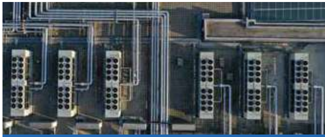
MEP & HVAC Projects
